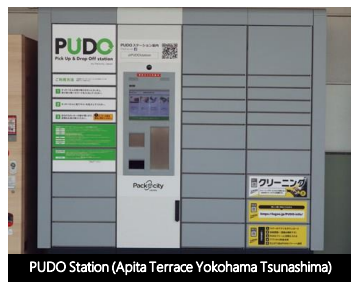
Installation of lockers to pick up products
