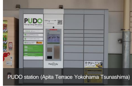
Installation of lockers to pick up products
