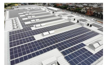
Kawamachi Yahagi Mall Power generation capacity: 302.40 kW
