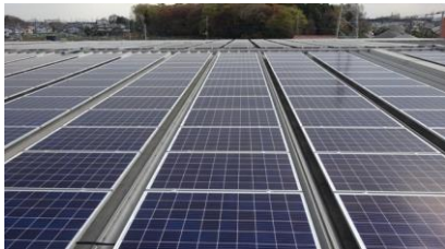
Unicus Ina Power generation capacity: 334.53 kW
