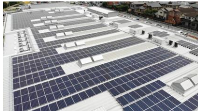
Kawamachi Yahagi Mall Power generation capacity: 302.40 kW
